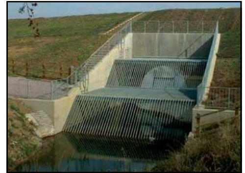
An exterior view of a vortex valve in Weedon Bec, UK
